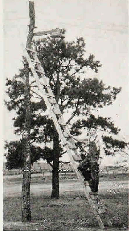
Pioneer 4-H linesman on duty, Edward Henry, who with his brother Jesse are installing most of the electrical equipment on their home farm.
